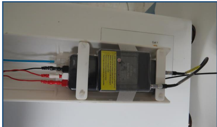
Fig 14: ERT module and battery positioned on a coil carrier
